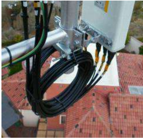
Figura 87 Cable jumper excedente
