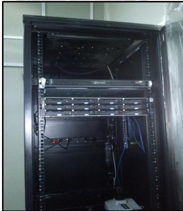
Figura 3.27 Gabinete 42U, NVR2100
