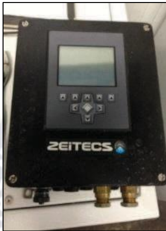
Figura 2.37: Panel de control Zeitecs
