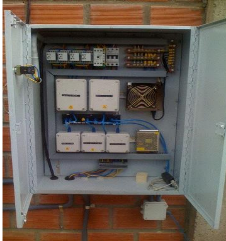
Figura 2.31: Tablero de control principal.
