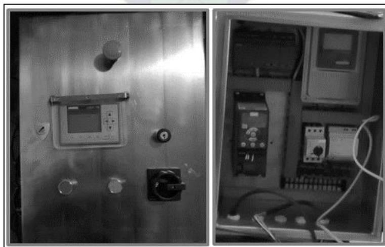
Figura 4.2 Tablero de control real.
